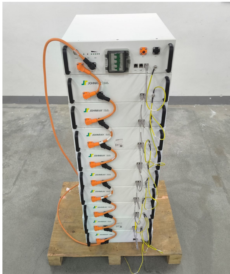
Front view of battery JRH51-S9
