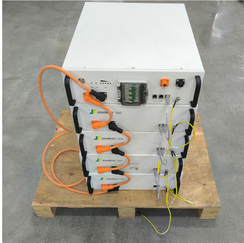
Front view of battery JRH51-S4
